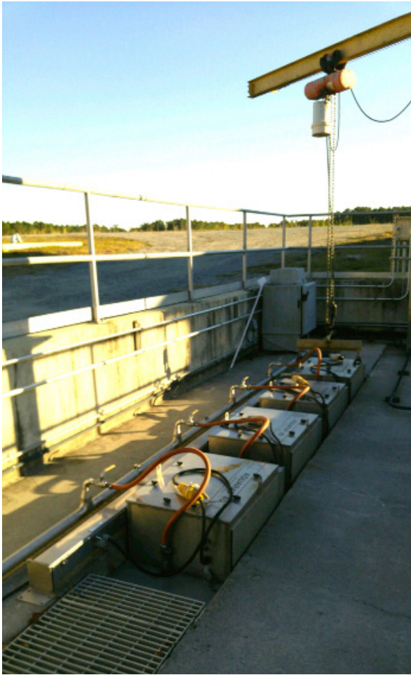
Existing 4 x 1 MGD low output modules
